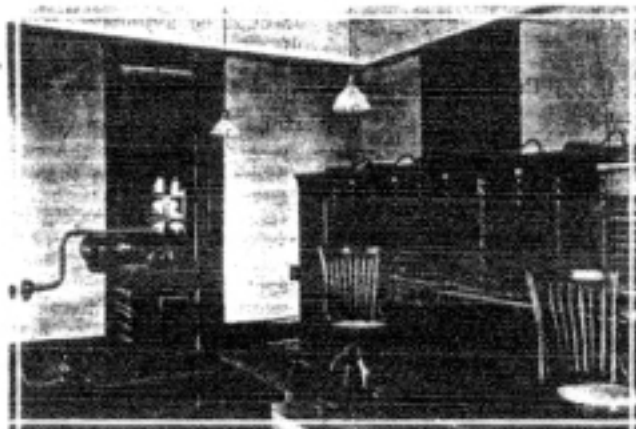
Main Switchboard and Chief Operator's Desk.
